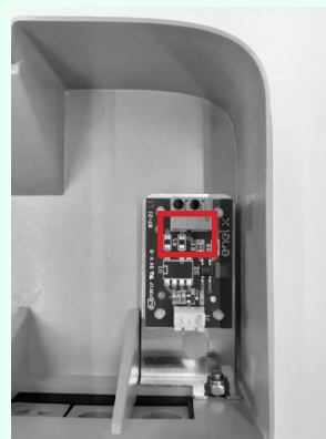
Clean contact on control board
